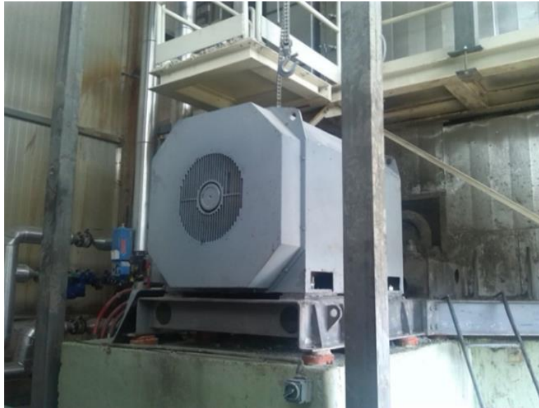
Fig. 1 HV electromotor in industrial plant
