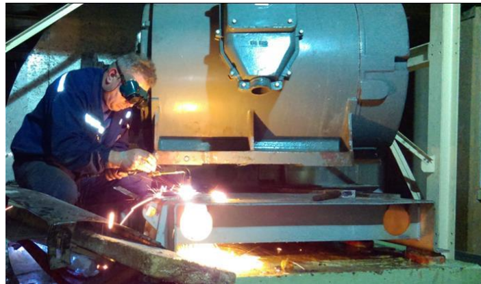
Fig. 8 Modification of the placement of the HV motor
