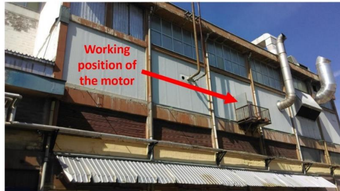
Fig. 5 Working position of the HV motor
