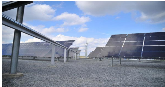
Fig. 2 Solar field in Belgorod region, Jakovljev district, 2010
